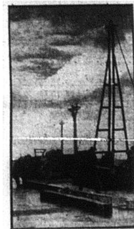
Corporation workmen repair sea defences after the gales. A breastwork is now being erected near Splash Point.
